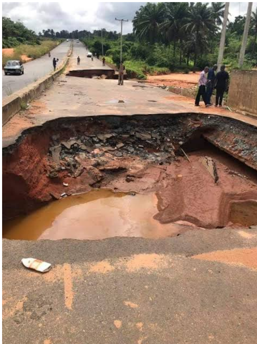
Figure 3. Bad roads in Nigeria.
